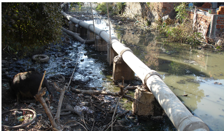
Sewage pipe and wastewater, Bhopal, India
