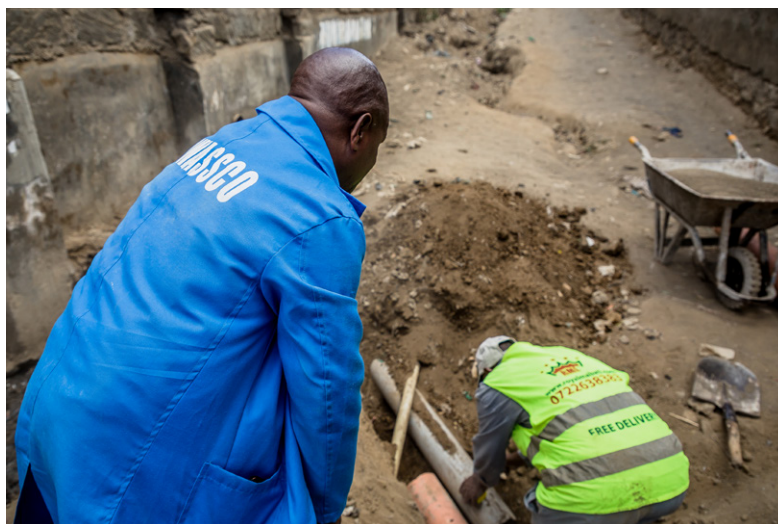
Image: Sewer line connection in Githima, Kenya. Credit: Brian Otieno.
