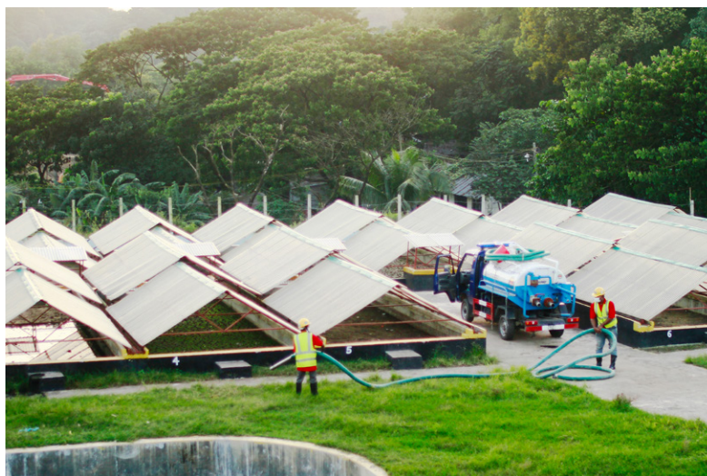
Image: Waste treatment plant in Chattogram, Bangladesh. Credit: Green Ink Media.
